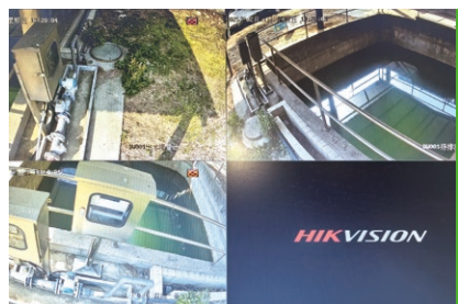
Wastewater monitoring system
