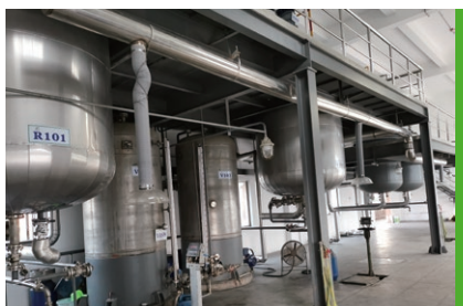
Workshops equipped with activated-carbon gas absorption system
