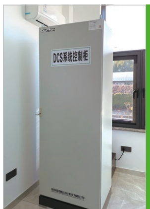
Distributed Control System
