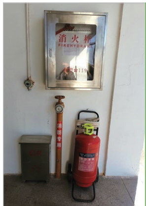
Fire-fighting equipment near workshops
