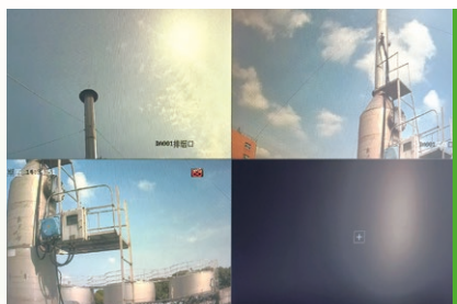
Waste gas monitoring system
